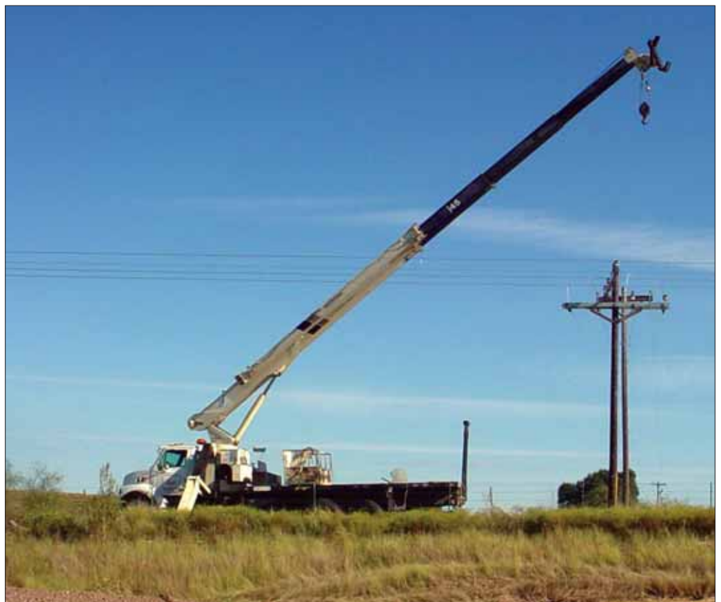
National Crane boom trucks help Chapman Construction install power transmission lines in remote locations.
