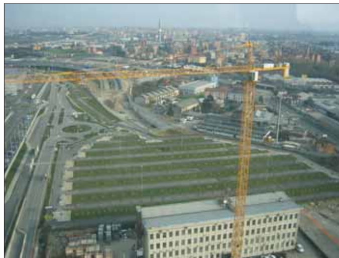
One of CMB's tower cranes in the Milan area working with a Manitowoc Crane CARE camera system.
