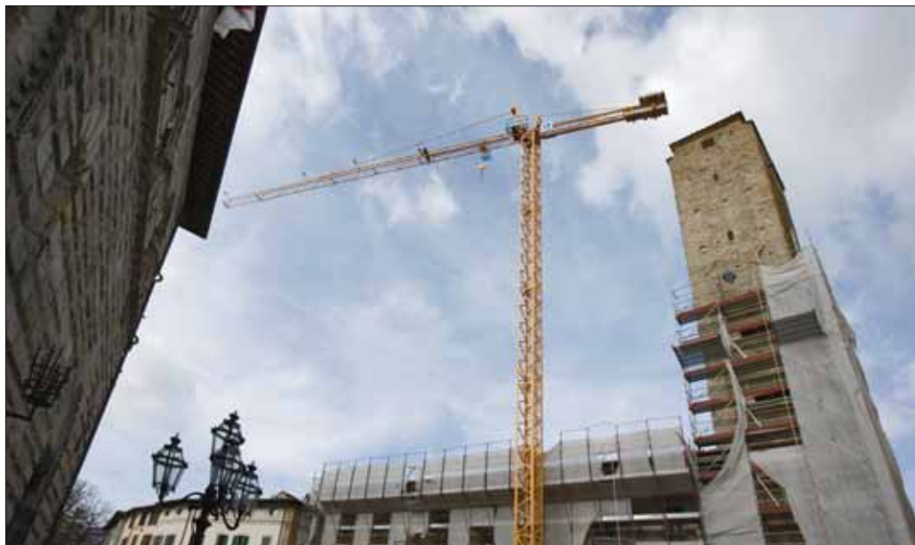
A Potain MC 68 C helped restore the Bishop's Episcopal Palace in Citta' Di Castello, Umbria, Italy.
