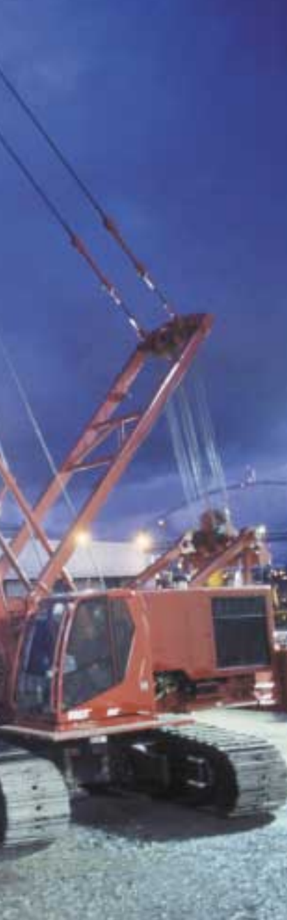
A Model 1015 at work in Portland, Oregon, US using a Leffer slurry wall grab.
