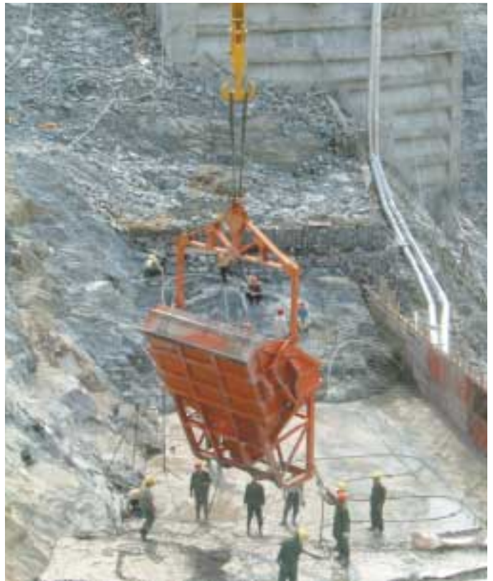
Workers position one of the enormous concrete buckets handled by the Potain tower cranes.
