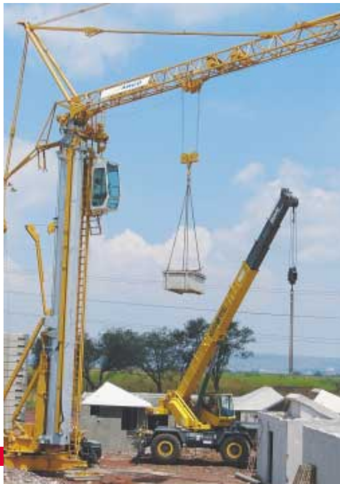
Grove and Potain products from Tracsa work side-by-side on a housing development site in Mexico.
