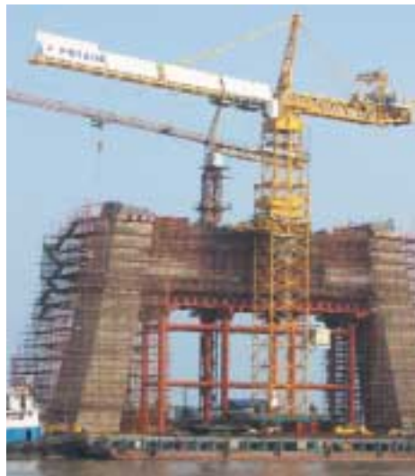
One of the Potain MD 3600 units at work on Nanjing Bridge #3. The cranes are the largest ever produced by Potain.
