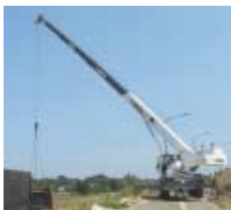
One of Aertssens' Grove RT600E units at work on the new high speed rail link between Antwerp, Belgium and Amsterdam, The Netherlands.
