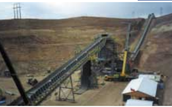
The crane was used to help construct a 15 km (9.3 mile) long conveyor system.
