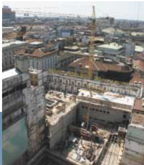
Potain cranes are aiding construction work at the Theatre Hall and Scenic Tower.
