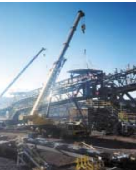
The crane was required to work seven days a week, spending two months in total on site.
