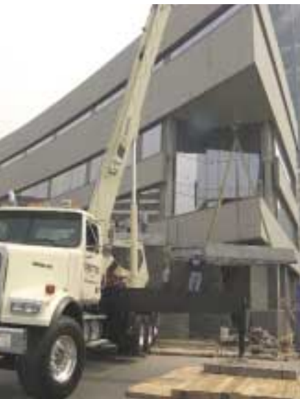
An 1800 series National Crane lifting a piece of structural steel at the Jewish History Museum in Battery Park City, New York. The 36 t (40 USt) capacity crane is owned by Metro Rigging of Huntington Station, NY.
