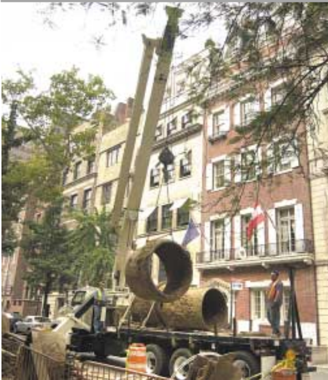
A 900A series National Crane boom truck removes sections of pipe as part of a utility project on Manhattan's east side near 69th Street and Madison Avenue. The 23.5 t (26 USt) crane is considered a true workhorse in the National line because of the 47.5 m (156 ft) tip height it can reach and because it has a large deck surface for carrying equipment. The crane is owned by Halcyon Construction of Pleasantville, NY.
