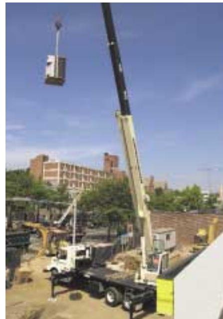
A National Crane 1300 series boom truck lifts air conditioning units onto the roof of a bank under construction in White Plains, NY. The 27 t (30 USt) capacity crane can reach a tip height of 49.3 m (162 ft) tip height. The crane is owned by AJ Cianciulli Inc of Yonkers, NY.
