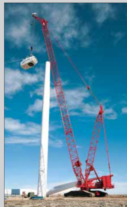
The cell on this wind turbine weighs 95 US t (86 t) with rigging.
