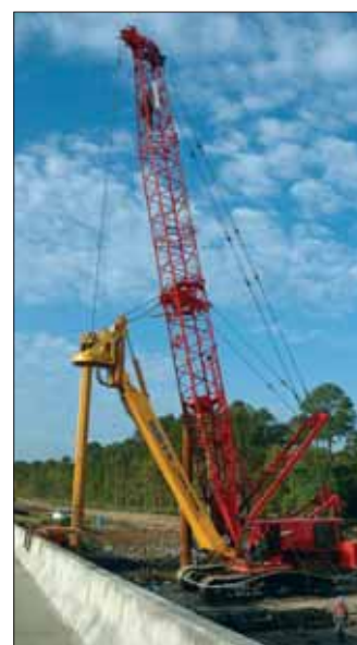
A barge-mounted Manitowoc Model 1015 helps with a replacement bridge project in Brunswick, Georgia, US.
