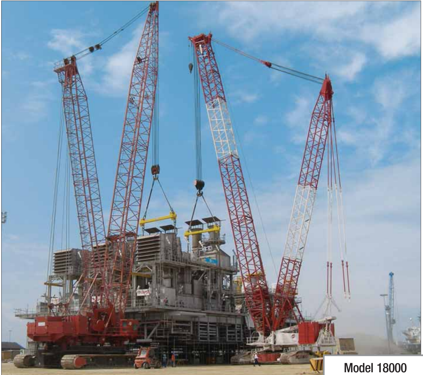
The Model 18000 worked with older Model 7000 and Model 4100W cranes belonging to the main contractor.
