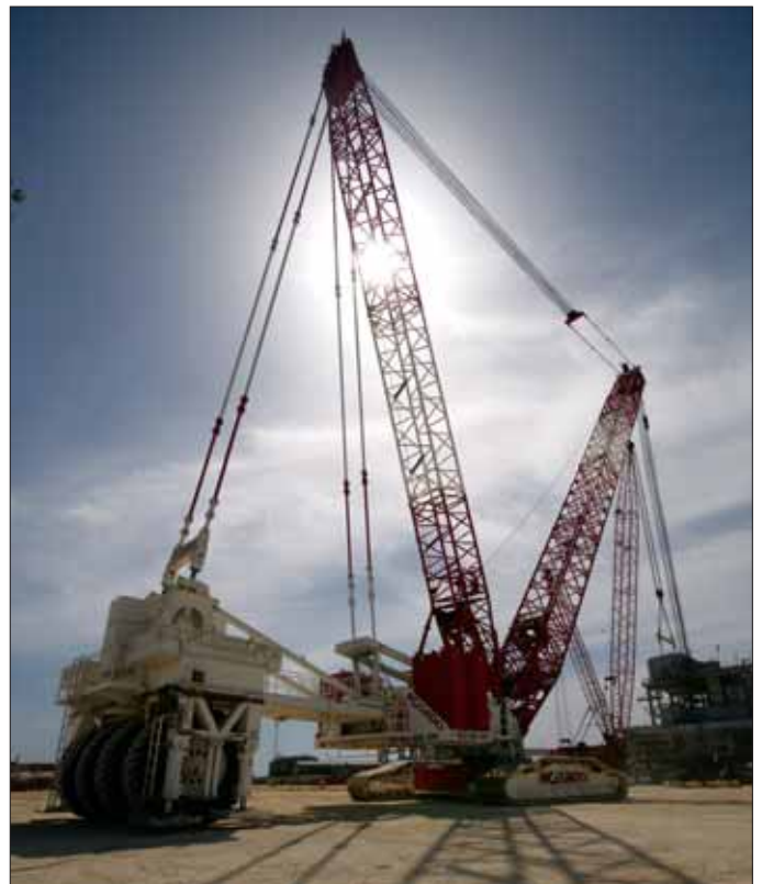
The capacity-enhancing MAX-ER attachment added 210 t (231 US t) of counterweight to the Manitowoc Model 18000 working in Spain.
