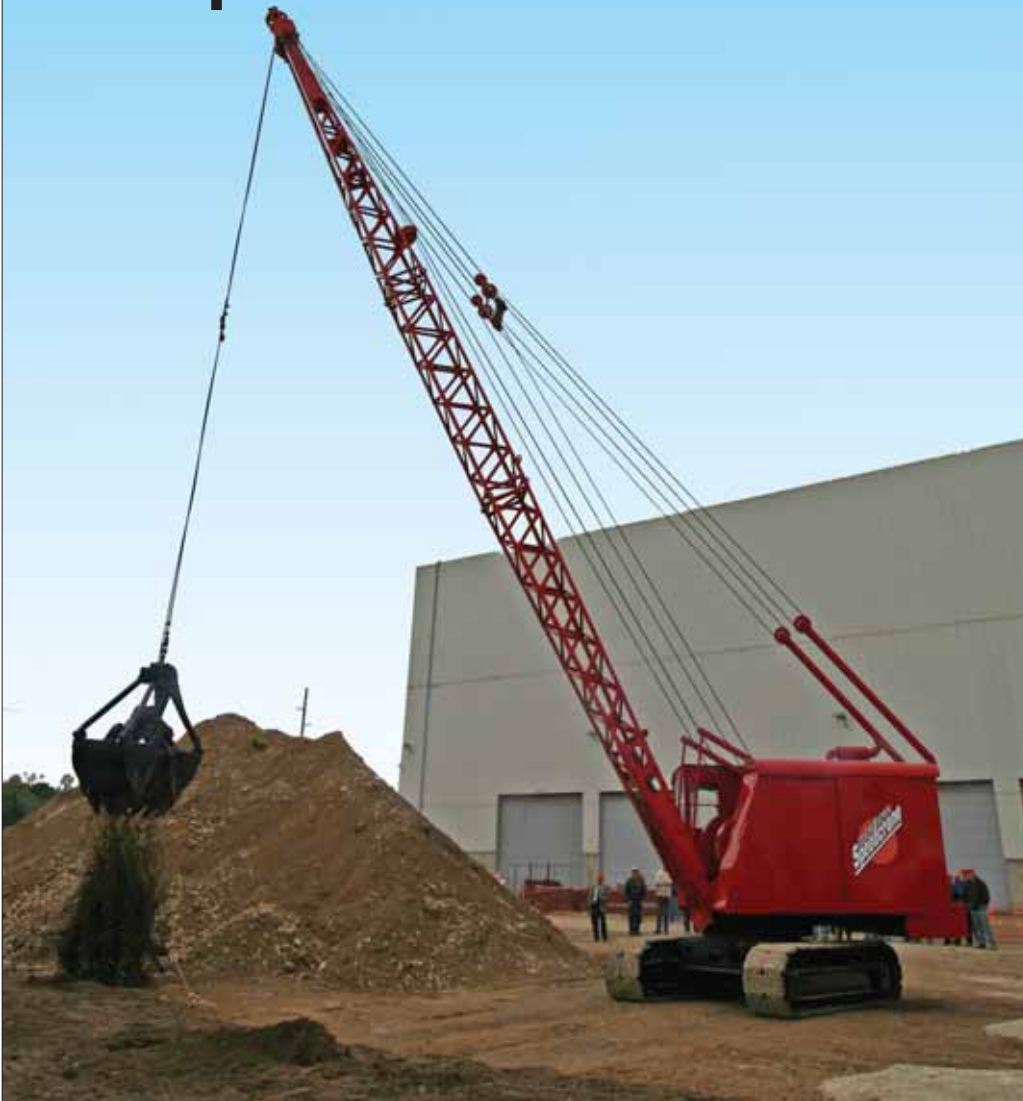
A 1941 Manitowoc Model 2000 Speedcrane, restored by Manitowoc employee Dick Vraney, broke ground on the expansion project in Manitowoc, Wisconsin.
